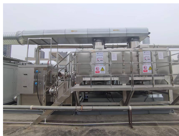
活性炭吸附浓缩+CO催化燃烧炉
